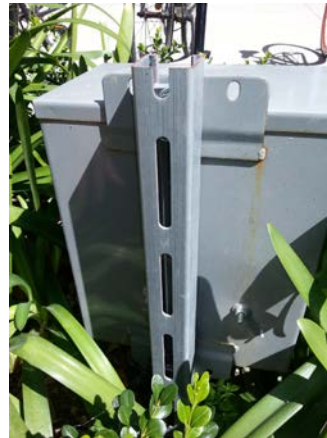
Enclosure on Unistrut in Planter
