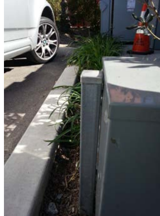
Enclosure on Unistrut
