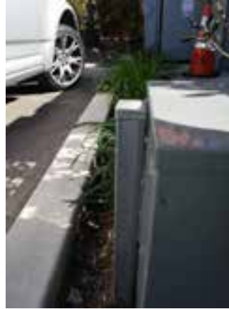
Enclosure on Unistrut
