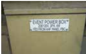
Labeling for Event Power Box
