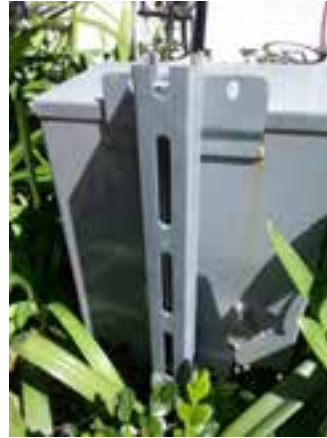
Enclosure on Unistrut in Planter
