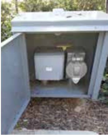
Lockable Enclosure with Outlets
