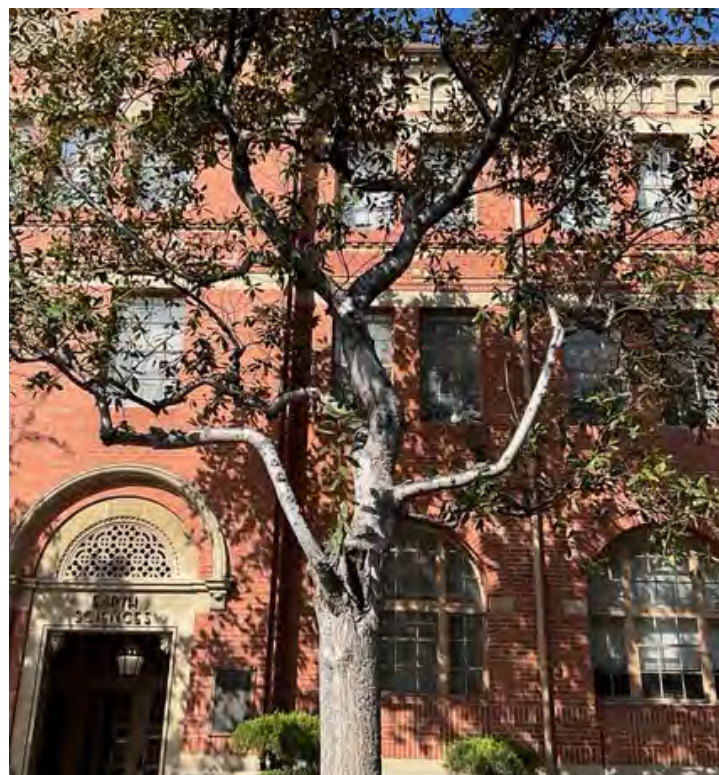
W09 Magnolia: To be Removed Within 5 Years Tree Decaying, With Weak Branches
