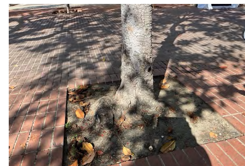
Compacted Soil Within Tree Well
